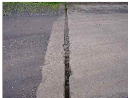
Figura 4. Junta sin sello y cubierto con tierra Figure 4. Joint lacking of pier ring, covered with earth
