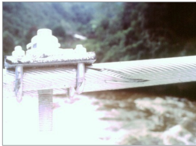
Figura 40. Catenaria principal con falla en alambres Figure 40. Main catenary showing wires failure
