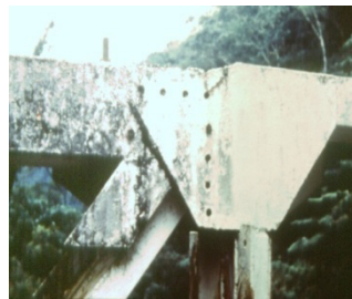
Figura 38. Falta de pernos, problemas de vibraciones Figure 38. lack of bolts, vibration problems
